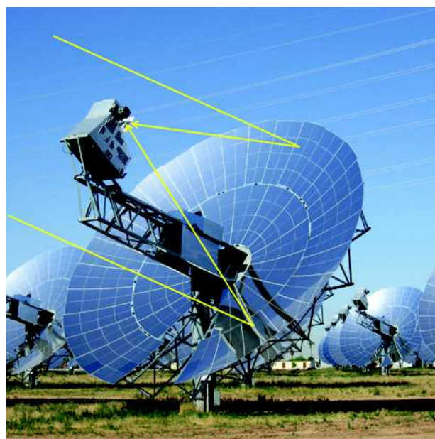
C: Dish Stirling system. Maricopa Solar Plant, SunCatcher
