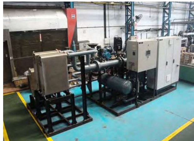
Fig. 6: Indigenously developed 100 kW e power skid
