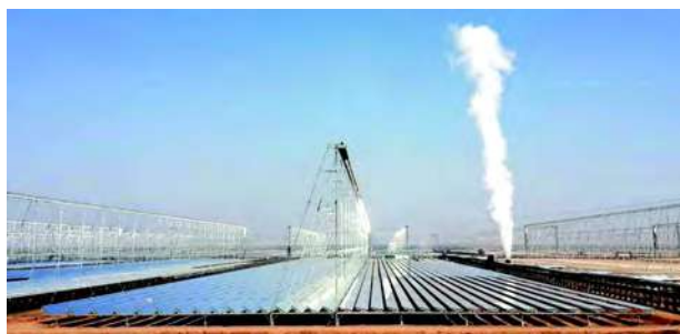
B: 125 MW solar thermal plant of Reliance (Areva, Dhursar)
